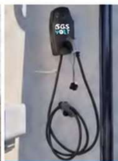
OCPPEV Charger in Azerbaijan
