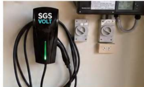
OCPP EV Charger in Brisbane, Australia
