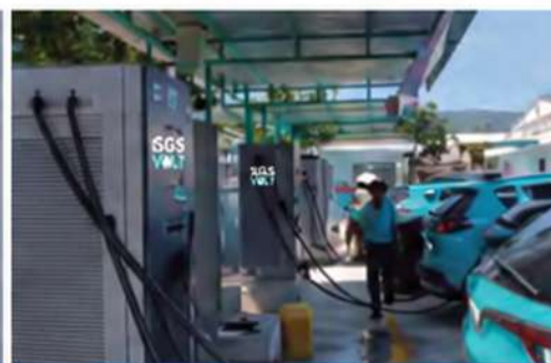
2 Guns DC EV charging stations with XE TAXI in Vietnam
