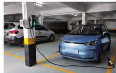
EV Chargers Installation in Brazil
