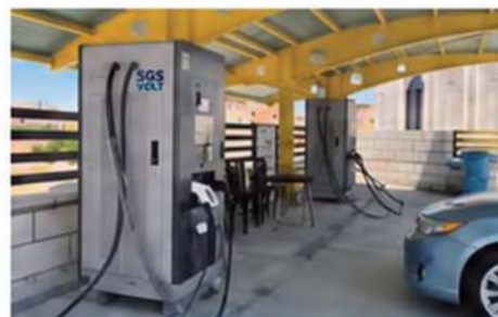
2 Guns DC EV Charger 120kW in Jordan
