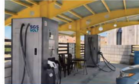
2 Guns DC EV Charger 120kW in Jordan
