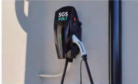
OCPP EV Charger in Azerbaijan
