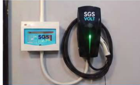
OCPP EV Charger in Myanmar
