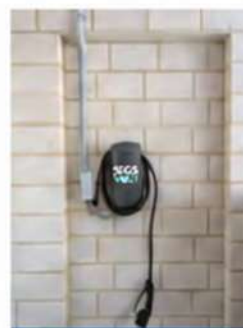
AC EV Charger in Perth Australia
