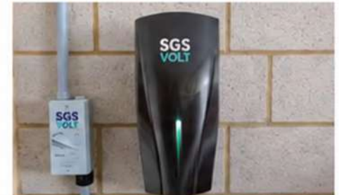
AC EV Charger in Perth, Australia
