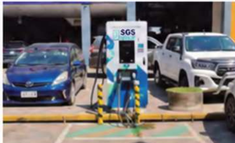
2 Guns 40kW DC EV Charger in Fiji
